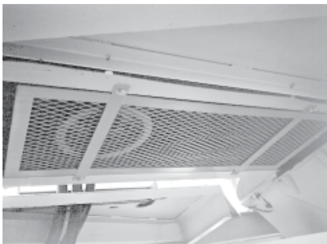
Properly installed belt guard
