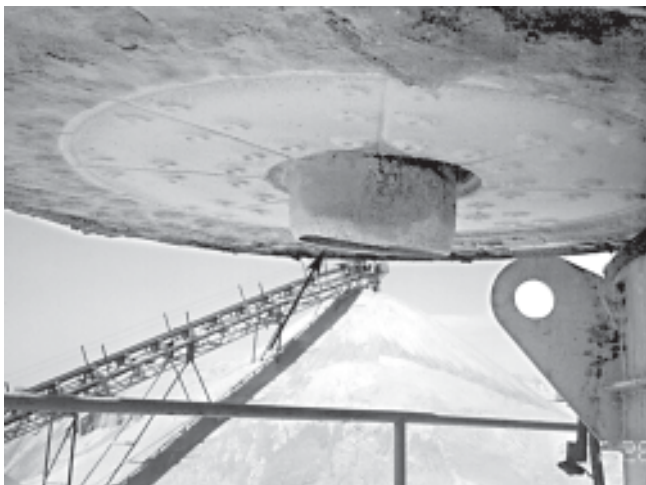
Non square feed tube liner improperly directs material into the rotor. This results in excess tube flange and upper ramp liner wear.
