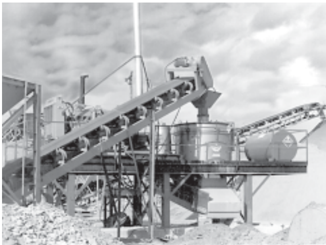
Frame mounted on a concrete slab
